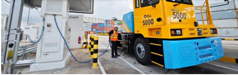
PSA hydrogen refueling station and fuel-cell electric prime mover vehicle (Image: PSA Singapore)
