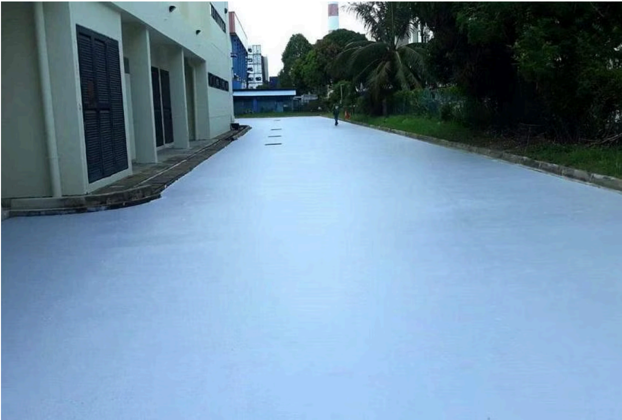
Pavements of an industrial area coated with the cool paint. PHOTO: NTU
