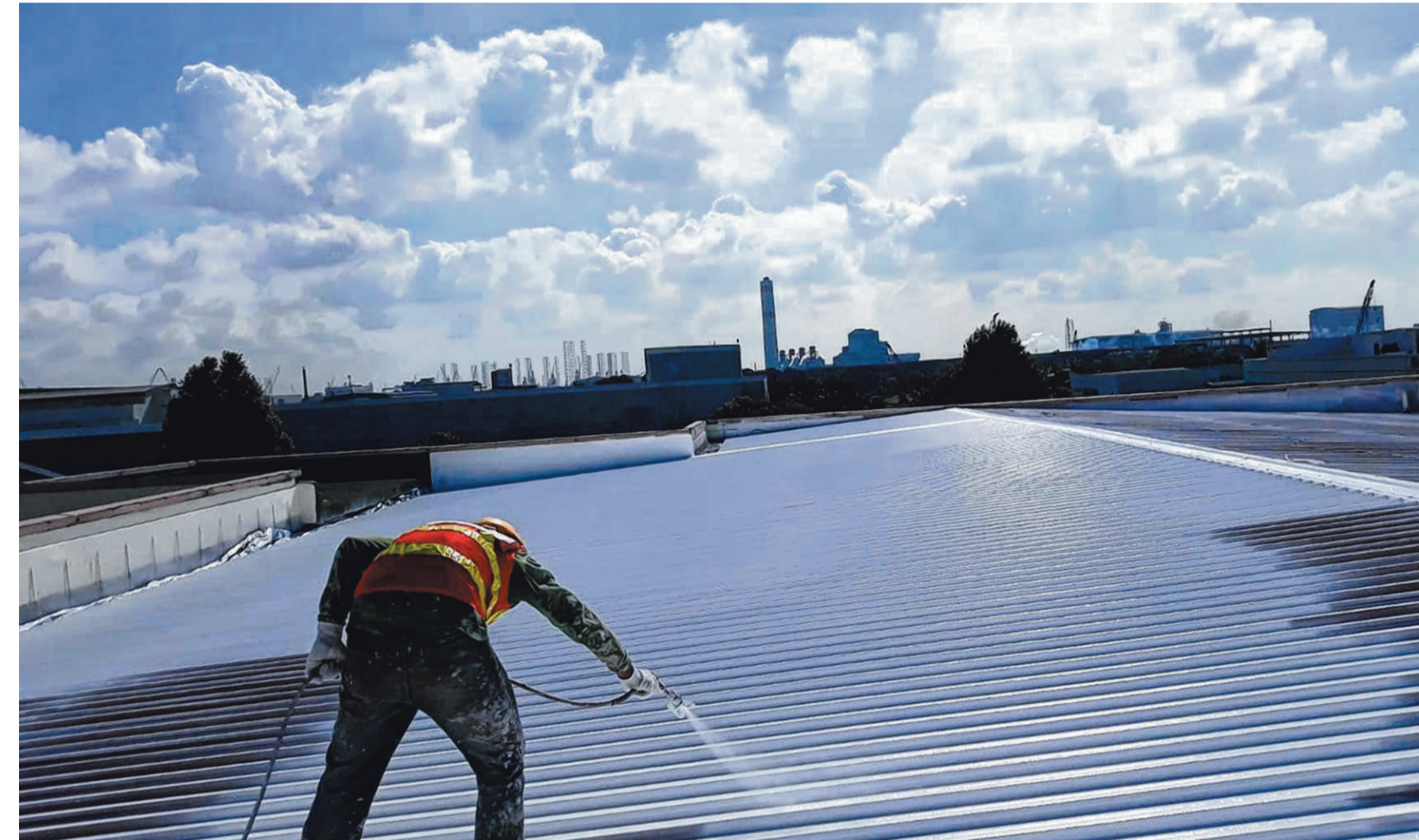
A worker spraying cool paint on the roof of an industrial building. In a Nanyang Technological University experiment done between 2018 and 2019, two industrial buildings and the road between them were coated with the paint, which contained a pigment that is good at reflecting sunlight. PHOTOS: NTU SINGAPORE
