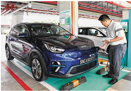
Once electric vehicle users register their vehicle with the GoParkin mobile app, they will be able to use the app as a one-stop platform to find available parking spots, charge their vehicles and make cashless payment. ST PHOTO: SHINTARO TAY
