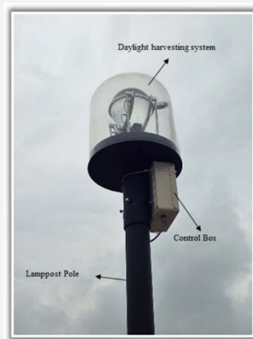
The 'smart' device to harvest daylight when installed on top of a lamp post pole. Image courtesy of NTU.
